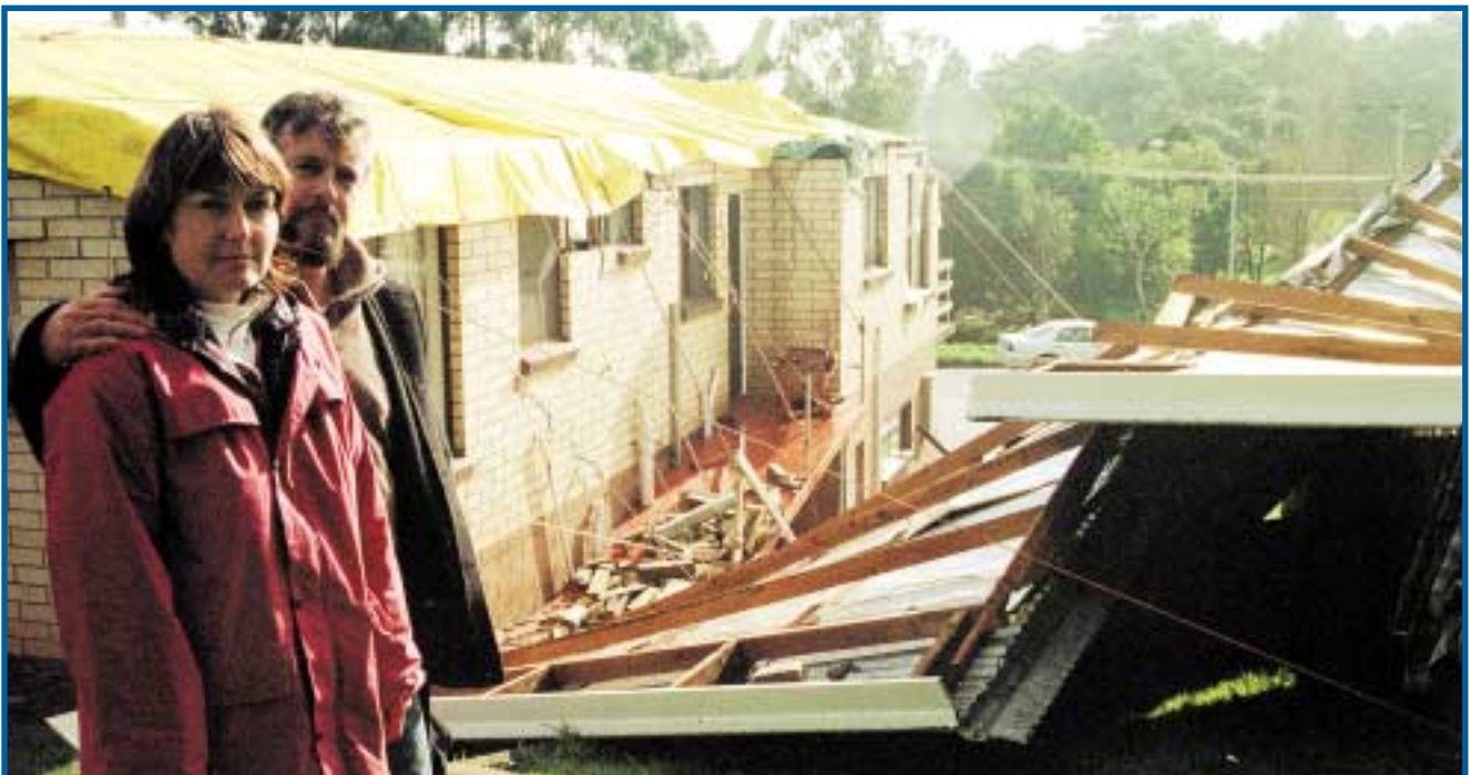
Storm damage at East Devonport, July 2000. Photo courtesy of The Mercury.
