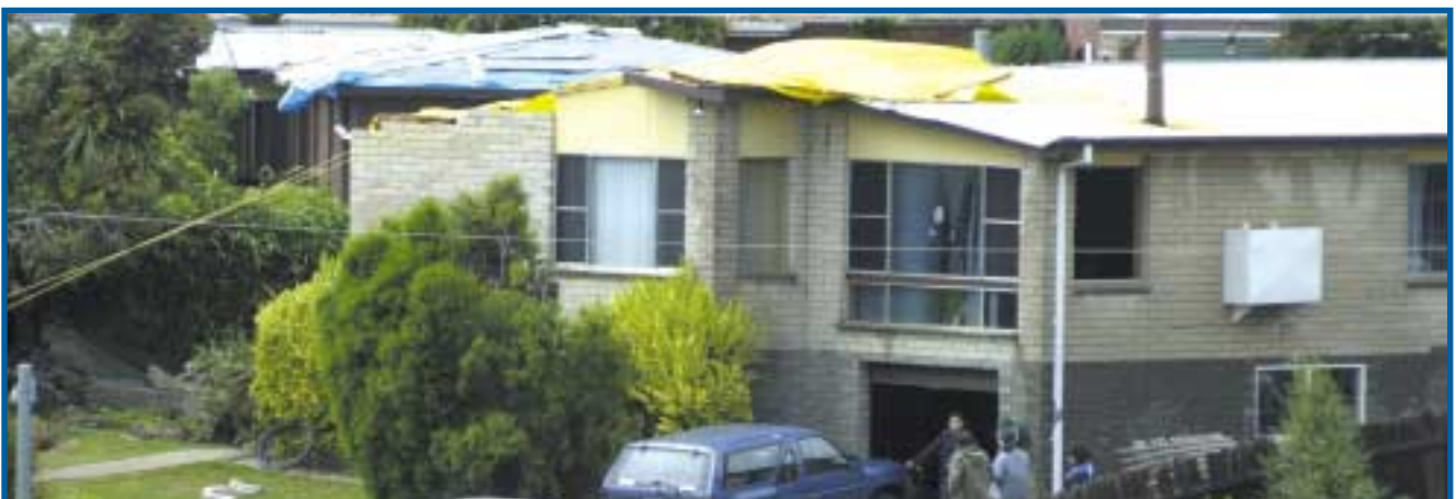
Storm damage at Summerhill, December 2001. Photo courtesy of The Examiner.
