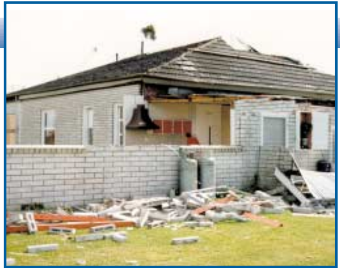
Tornado damage at Smithton, November 1992.
